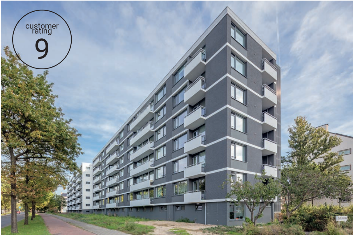
Renewal and major maintenance of Jolandaflat - From label E to A - Sustainability project Jolandaflat
